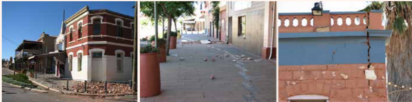
Figure 7: Damage from the magnitude 5.0 Kalgoorlie-Boulder earthquake in different structures located in Boulder. Photo source: DFES – Goldfields-Midlands.
