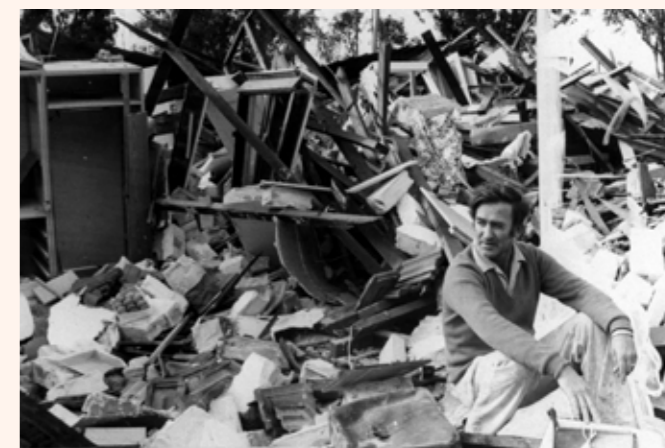
Figure 3: House damaged during the Cadoux earthquake in 1970. Photo source: © WEST AUSTRALIAN NEWSPAPERS LIMITED.
